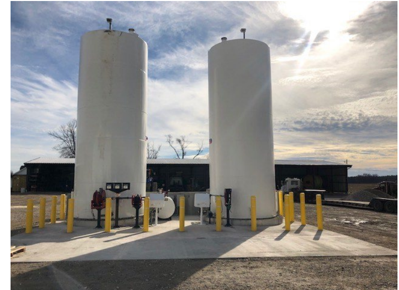
Two 20,000-gallon storage units.
